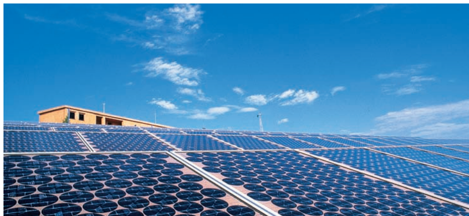
FIGURE 22.26 Silicon solar collectors are used on a large scale to harvest energy from the sun in this photovoltaic power plant located on one of the Tremiti Islands in Italy. (© Tommaso Guicciardini/Science Photo Library/Photo Researchers, Inc.)
